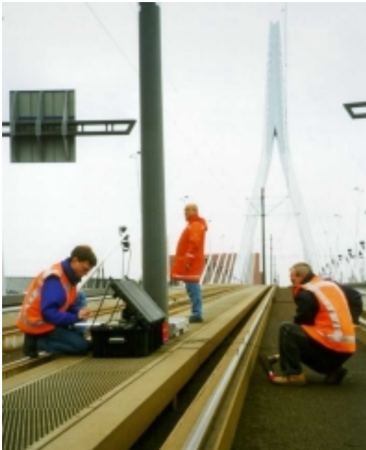
Fig. 3.3.1: Impulse hammer test on tramway track at the Erasmus bridge in Rotterdam
