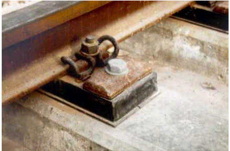
Fig. 9. Elastic rail support in track structure, Berlin
