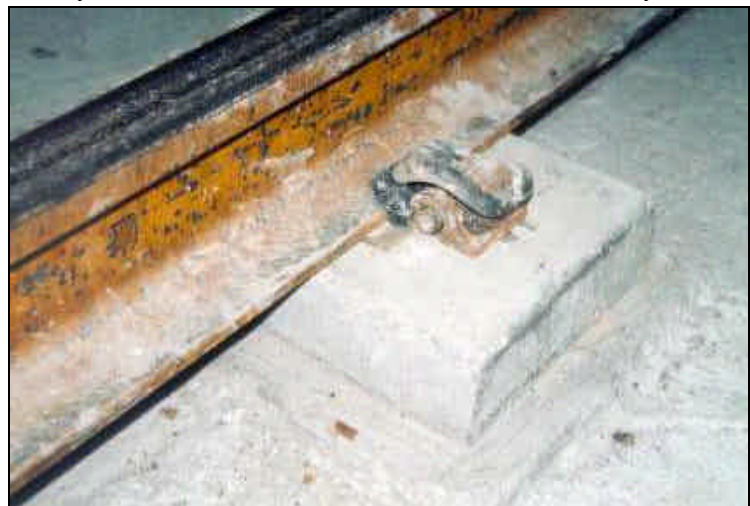
Fig. 7 Detail of Edilon Block System with Pandrol fasteners
