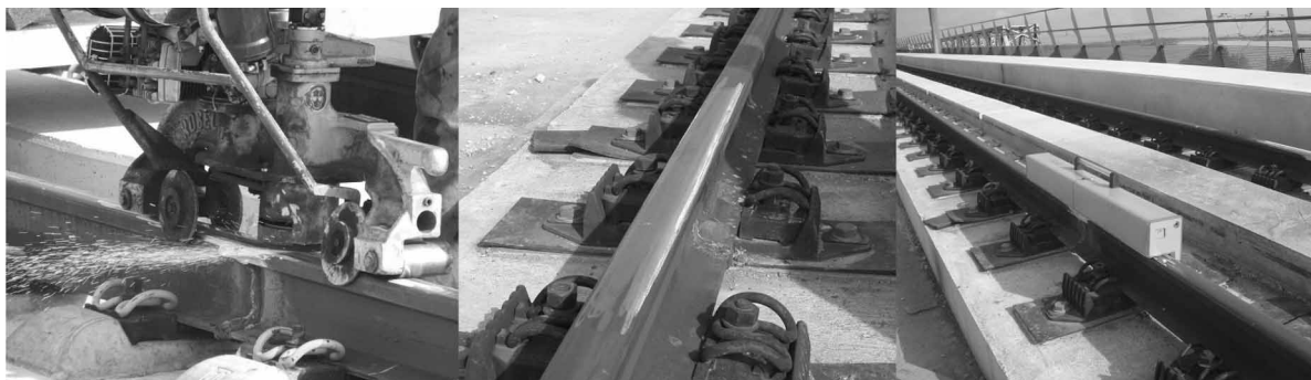
Fig. 21 Semi-mechanical grinding of the rail weld surface in longitudinal direction, ground rail, and electronic geometry measurement
